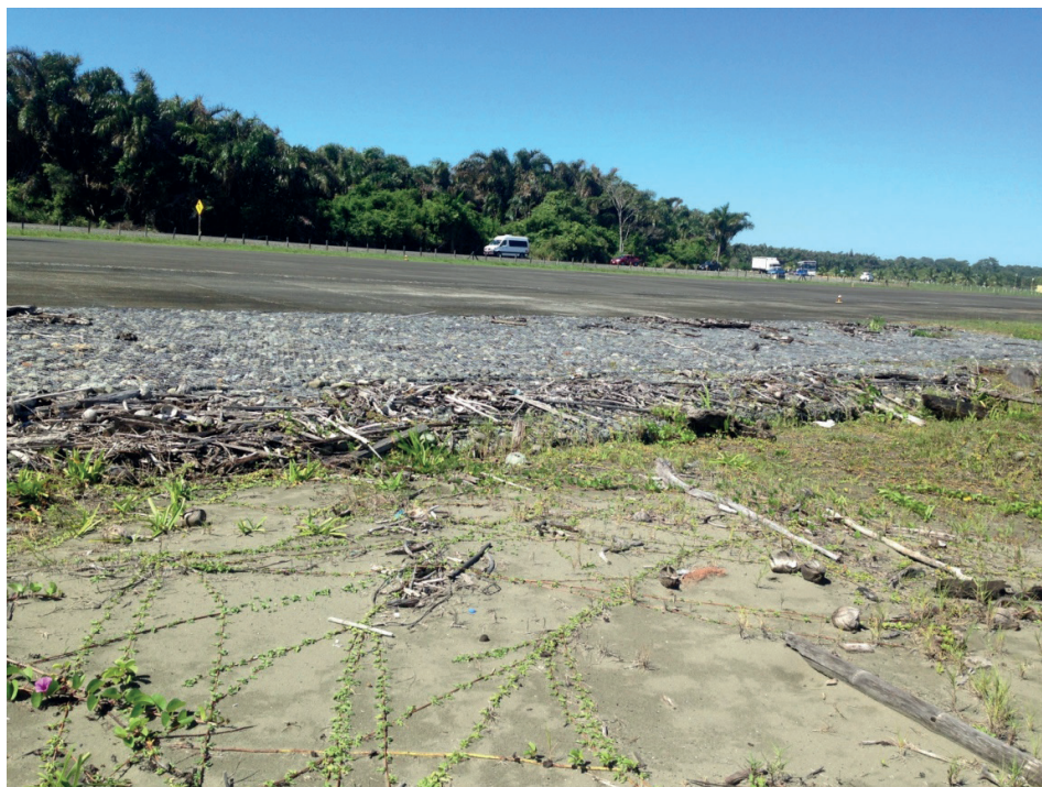
Figure 6. Stone and wire mesh covering on one side of the airport runway where erosion has made necessary such repair works.
