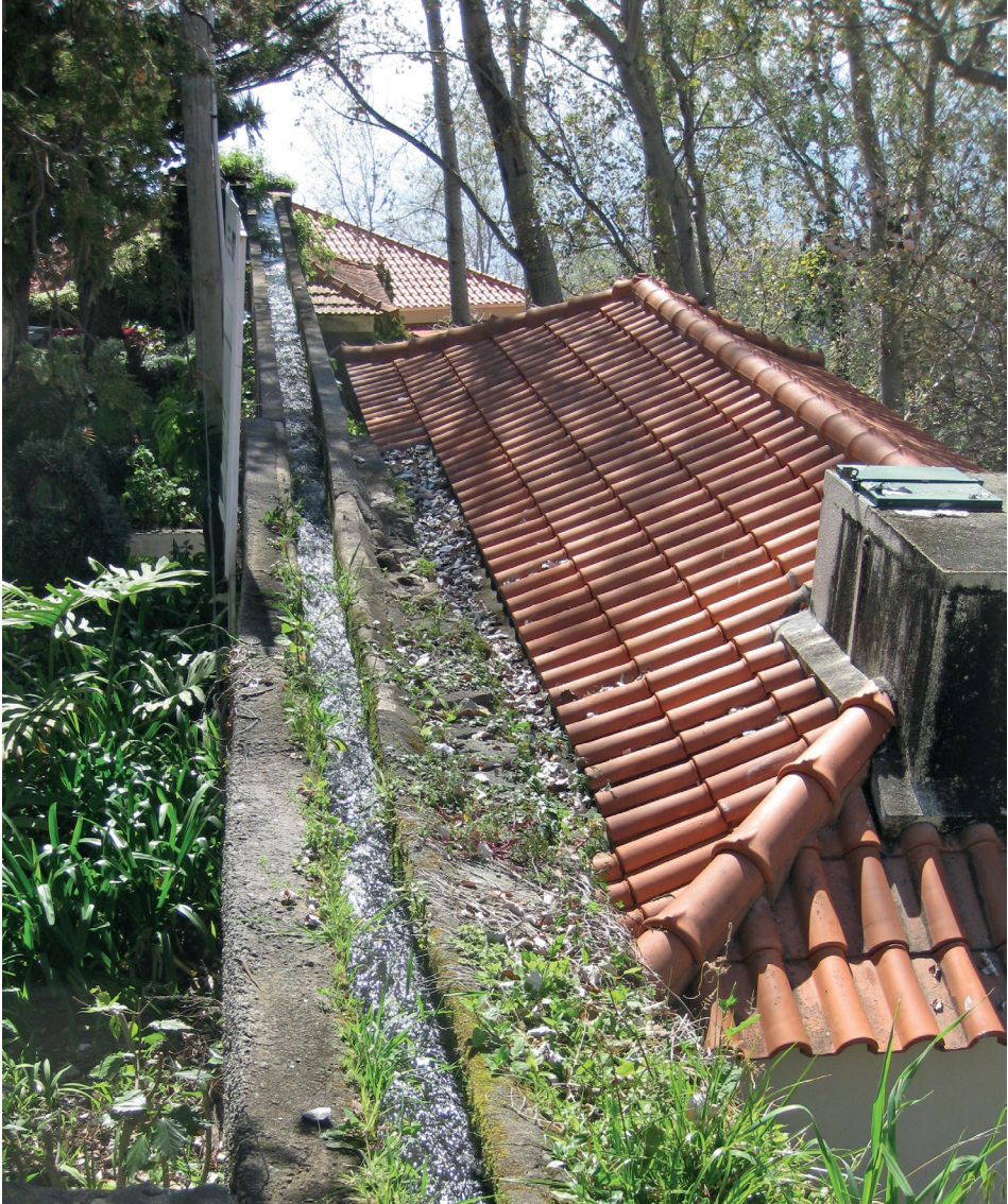
Figure 14. View along the top of the aqueduct that carries to the mill in Lombada. Compare this view with that in Figure 4.
