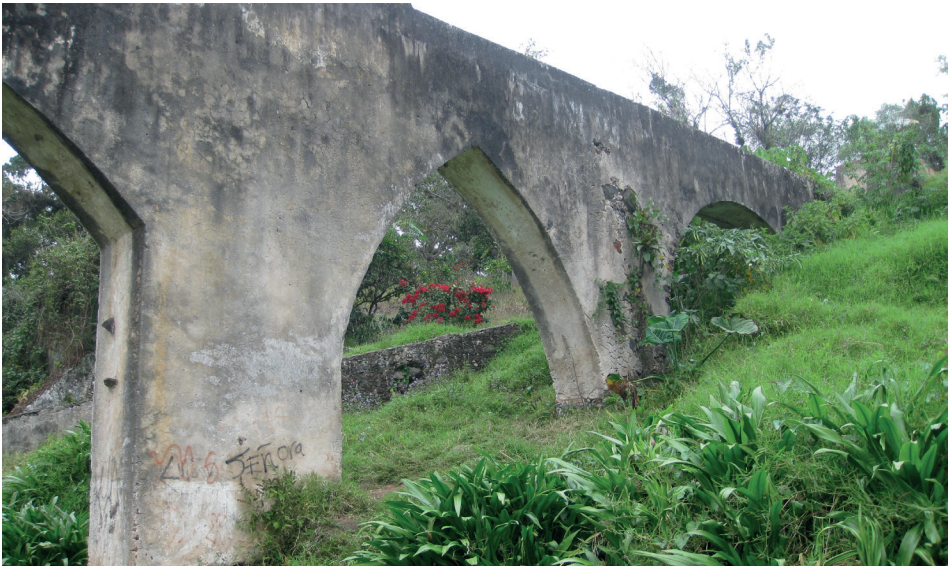
Figure 6. In addition to having a circular arch (right) this aqueduct is characterized by Gothic arches.
