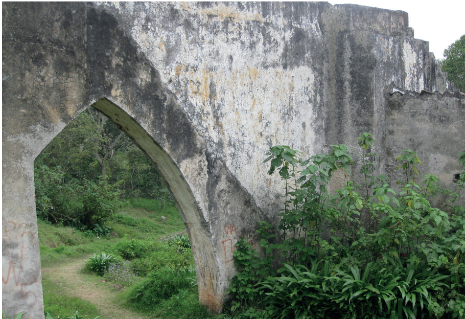
Figure 7. A view opposite that of Figure 6. Clearly evident are the widened pier/narrowed span, and the addition of a penstock.
