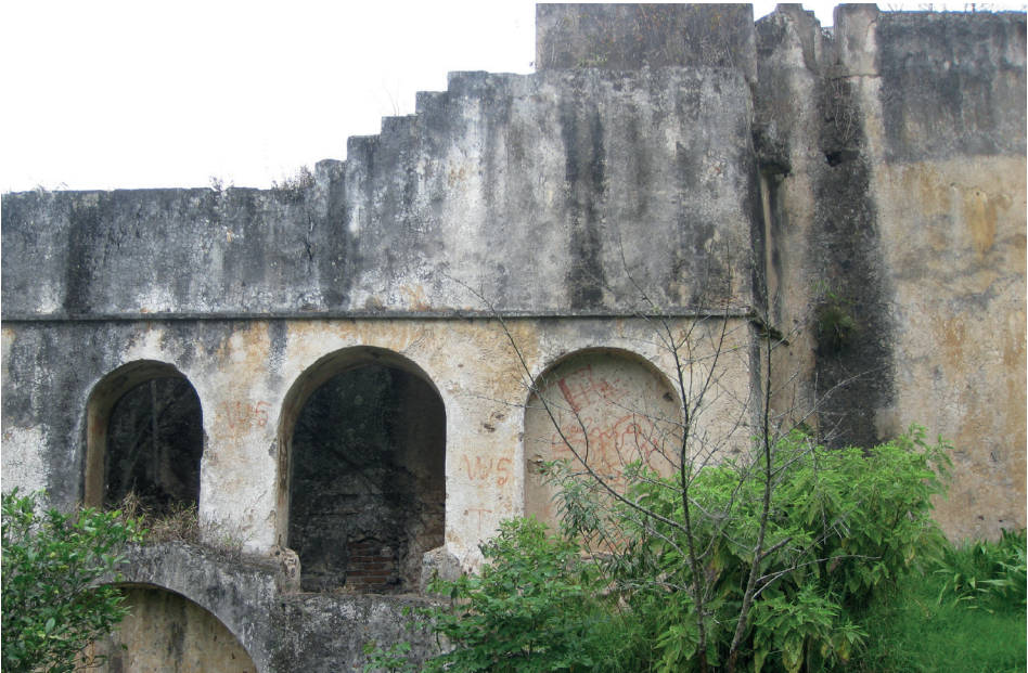
Figure 3. Profile view of the mill structure at Hacienda de Pacho. Water entered the mill through a channel in the upper right, dropped into a penstock behind the arch on the right, and turned a milling device below. Water exited the mill via a chase behind the lowest arch visible in the lower left.
