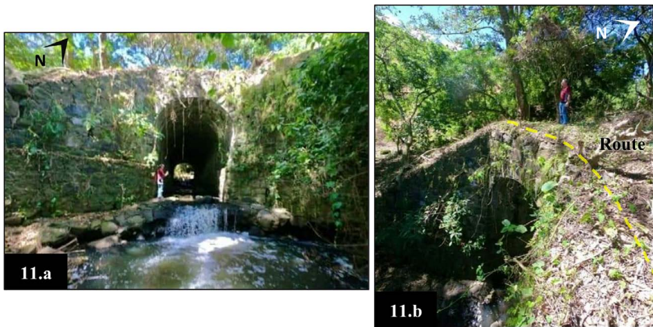
Figure 11. Site view of the bridge Puente de Bechee built in the study area, over the Púcares River (1.a), for the railway route overpass (11.b).
